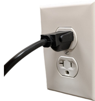
120VAC Receptacle (wired to on/off switch)
